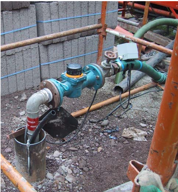
The wellhead at the UCC Arts Museum Building
